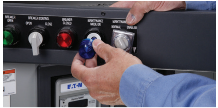
Mechanical servicing of Substations and switchgear (Chapter 12) include a verification of mechanical indicating devices, such as breaker status lights
