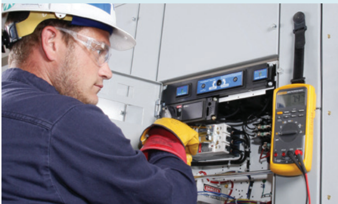
Motor control centers (MCC) are included in Chapter 28 of NFPA 70B. Requirements for MCCs include visual inspections, lubrication, mechanical servicing, and electrical tests.
